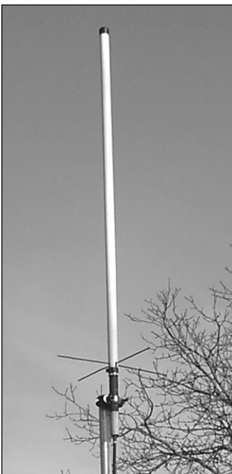
Figure 16.64: The finished antenna installed on a mast
