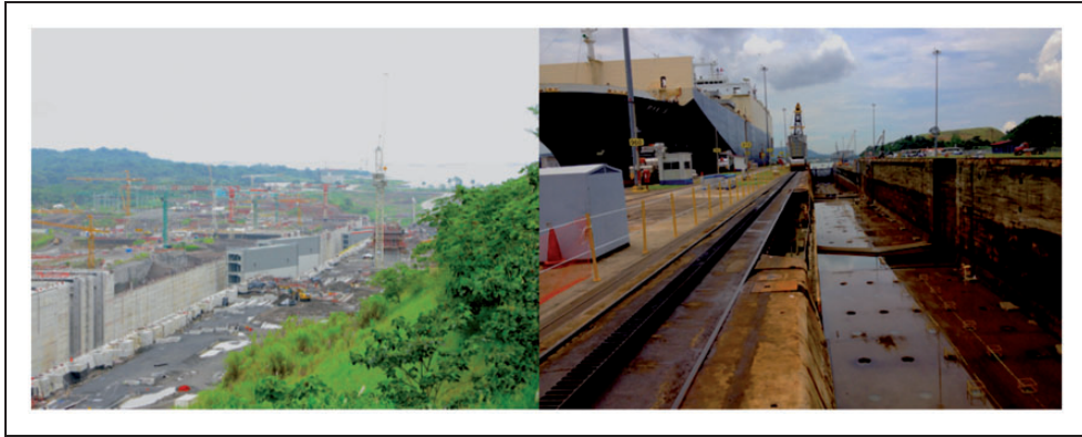
Figure 2. The Panama Canal expansion project (2006–2016) involved the construction of a third flight of larger locks to complement the two flights of original locks and the deepening of channels and harbors. The canal’s original locks (right) set the Panamax shipping standard. The new locks (left), shown here during construction in 2012, allow larger ships to transit and set the New Panamax standard. Photos by Ashley Carse.
